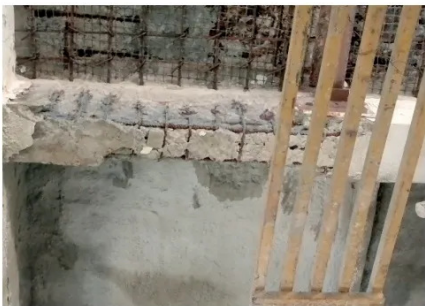
Fig. 1: Distress in structural element
